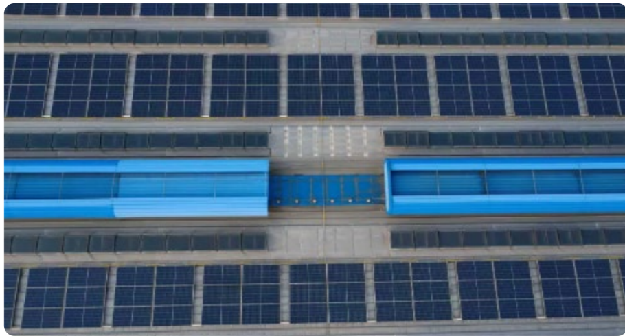
Picture of Photovoltaic Panels at Nantong Plant
