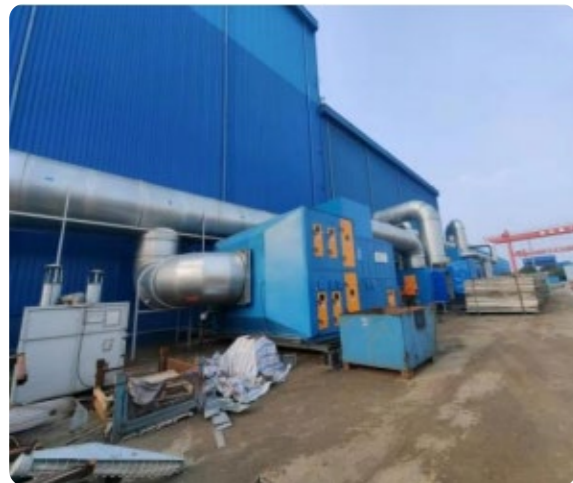
VOCs Waste Gas Treatment Facilities
