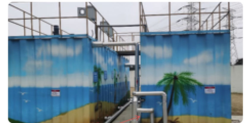
Picture of Wastewater Treatment Facility at Morimatsu's Nantong Plant
